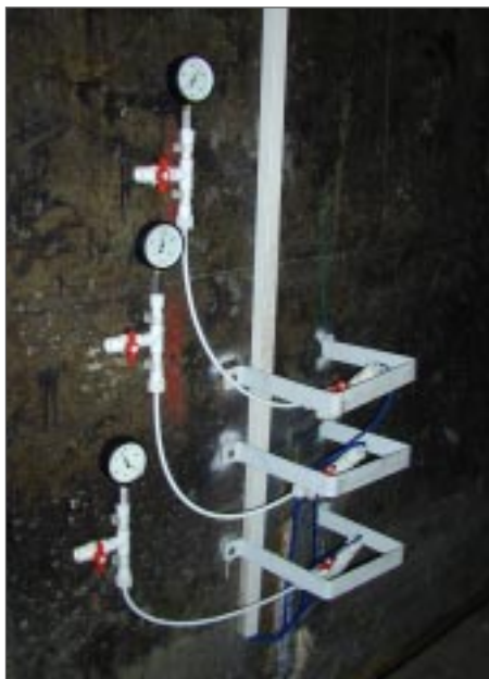
Measuring the water level with the piezometers Geokon model 4500S
